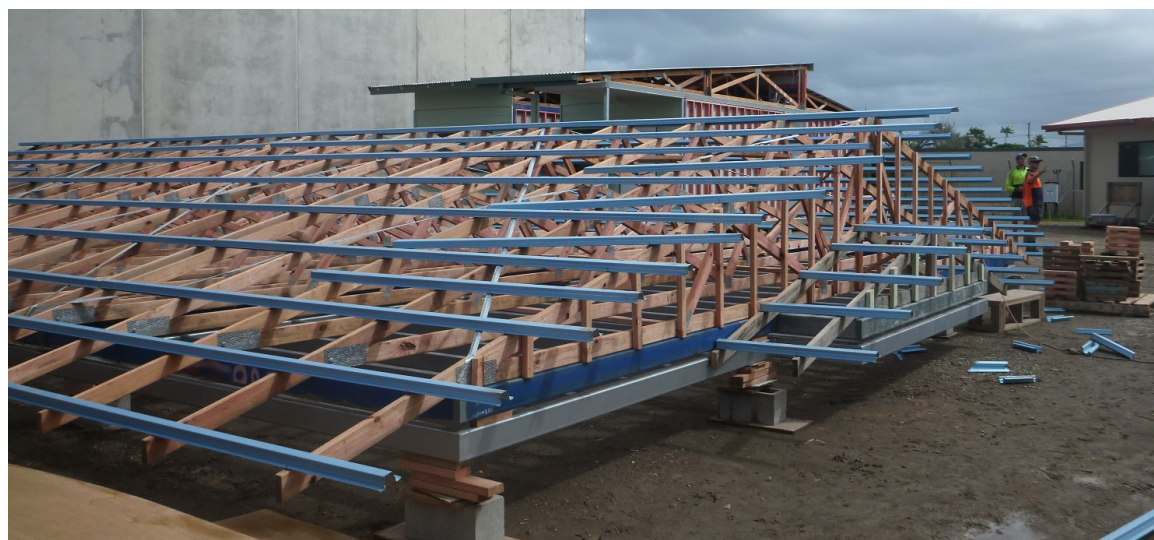
Prefabricating roof at ground level to eliminate work at height, Remote Building Solutions.
