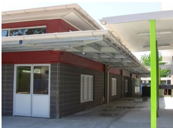
Perimeter path allows access for plant for safe maintenance. Photo: Education and Training Directorate.
